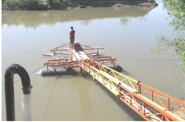
Figure 24: Micro hydropower station MHCF D4x1,5E installed on river Prut.
