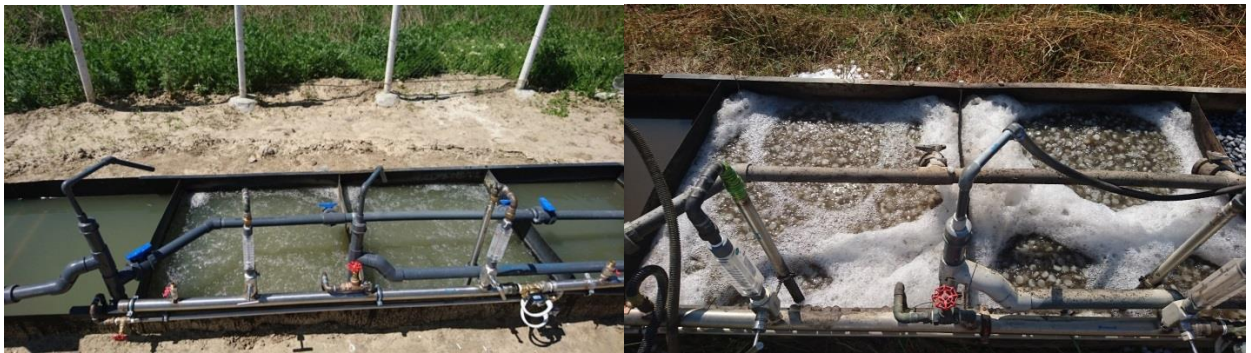
Fig. 2.3. Pilot wastewater treatment plant on which the experiments took place
