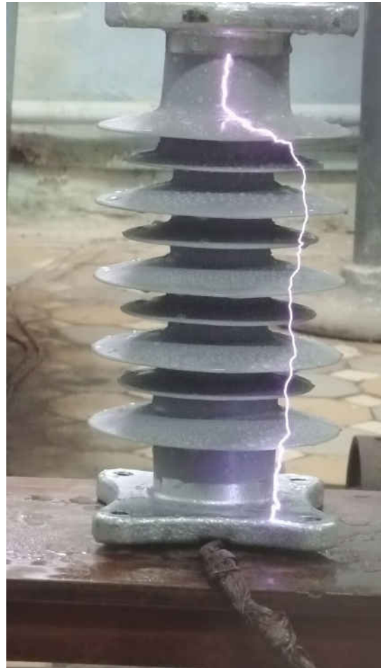
Fig. 9. Overlapping of the moistened insulator.
