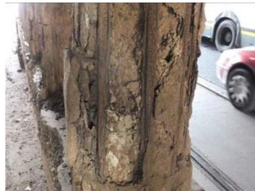
Figure 8. Degradations of the pillar support [6].
