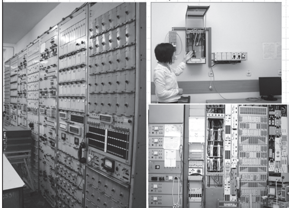
FRT. Laborator sisteme de transmisii optoelectronice - MOLDTELECOM
